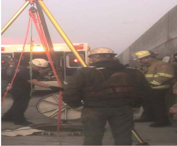
Pictured - Captain Jeran McCormick (Left) and Battalion Chief Jack Woodard (Right) work with surrounding fire agencies on the Hood Canal Bridge Confined Space Recue on 30 September 2009.
